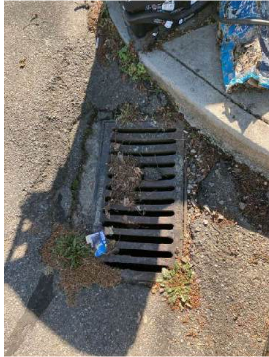
Hazelwood #2– Inlet on Westwood Circle with debris
