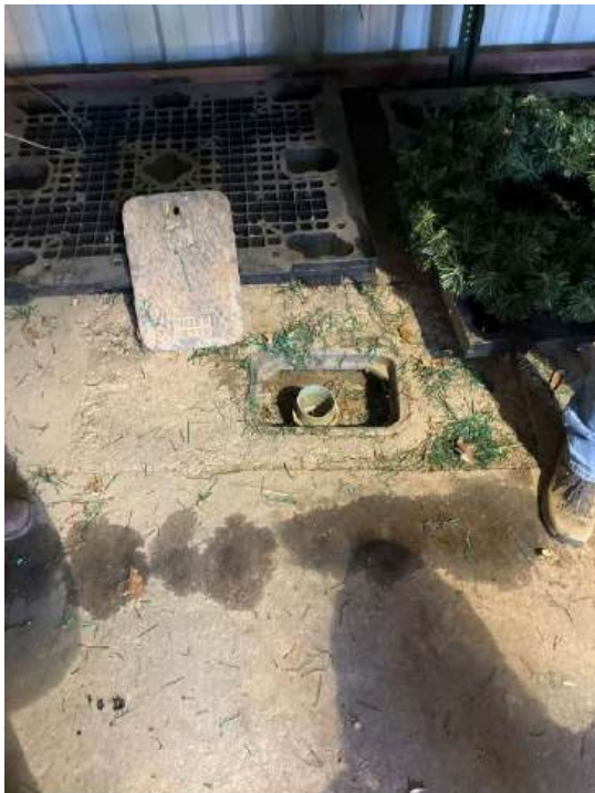
Public Works #3 – External Clean out Access
