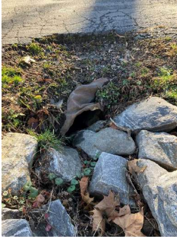
Greenway Rain Garden #4 – Compromised Culvert underneath driveway
