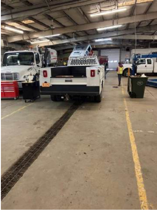
Public Works #1 – Floor Drain inside garage
