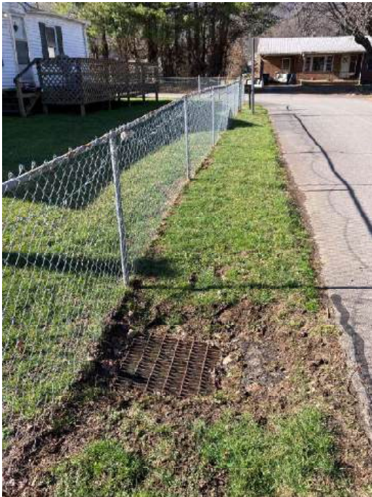
Hazelwood #3– Inlet on Westwood Circle that collects grass clippings
