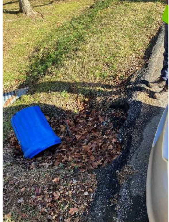
Fire Station #6– Gully erosion adjacent to pipe
