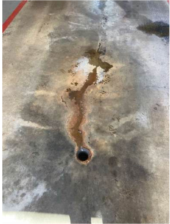
Fire Station #2– Parking Bay Inlet 2
