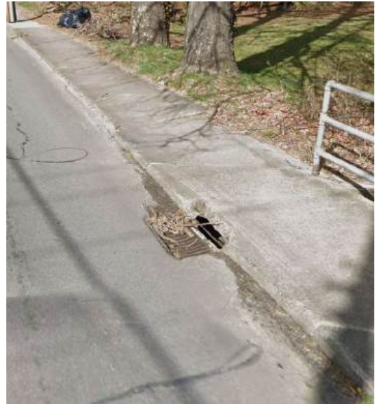
Fire Station #8– Brown St inlet on east side missing curb
